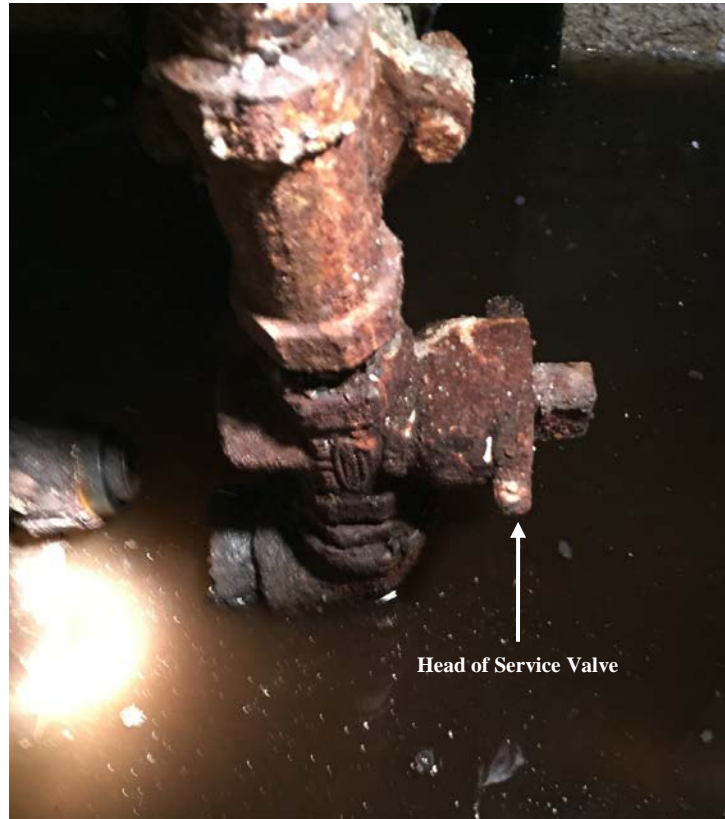
Photo 2 Gas Service To The Fire Building (Post Explosion)
