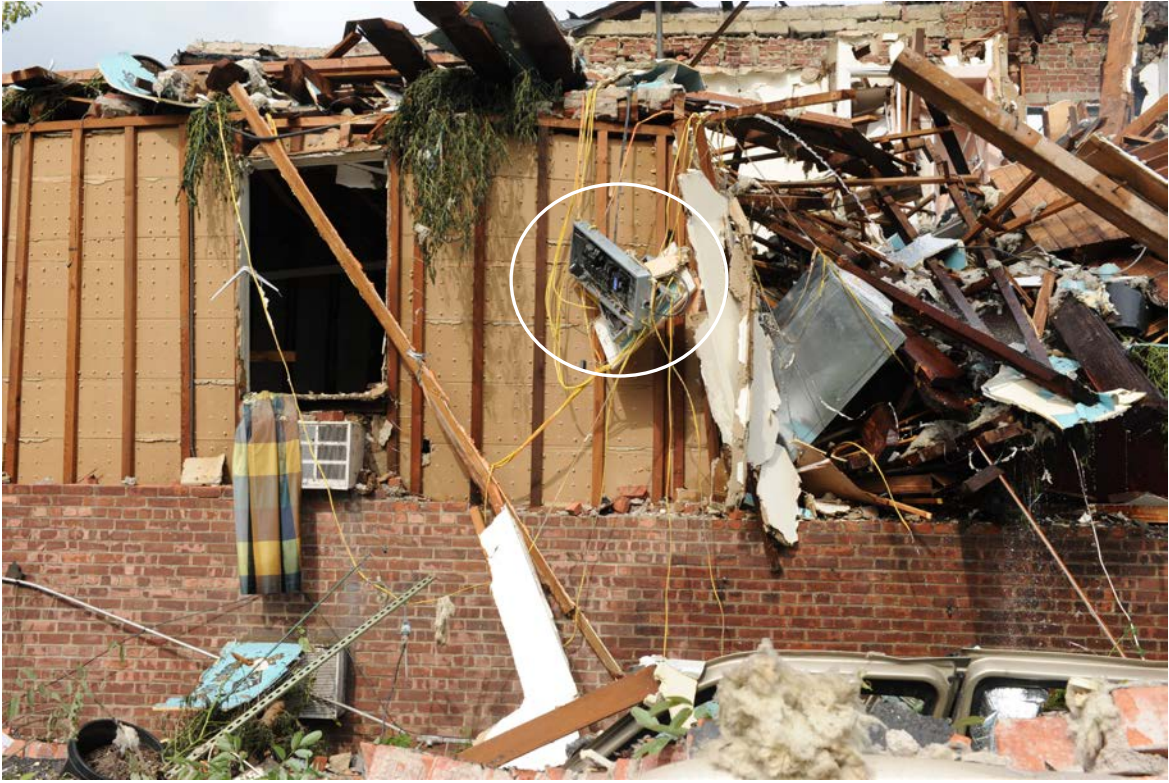
Electrical Sub Panel Illegally Installed on the 2 nd Floor
