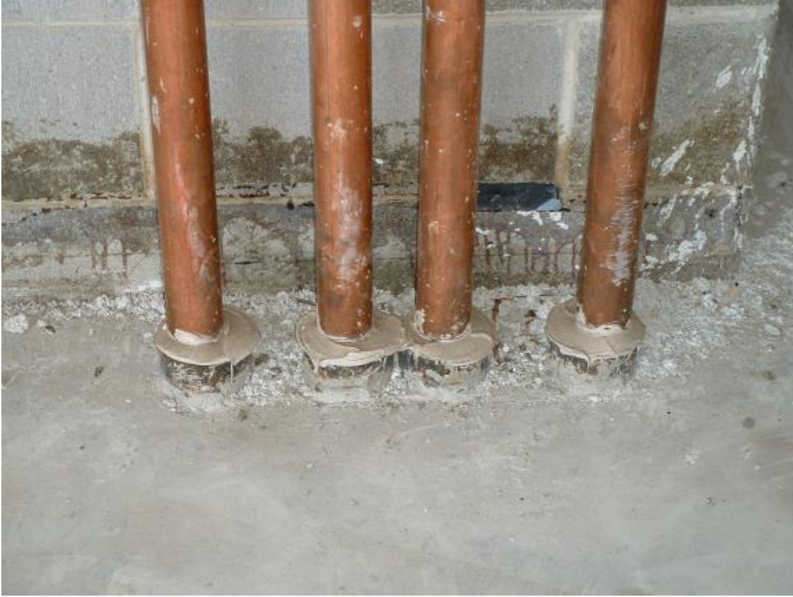
Photo 4 shows four pipes penetrating a two-hour-rated structural concrete floor, each with its own steel pipe sleeve. The space between the pipes and sleeves has been packed with mineral wool insulation; the tops of the sleeves have been sealed with cement grout; and the bottoms of the sleeves have been sealed with fire caulk.
